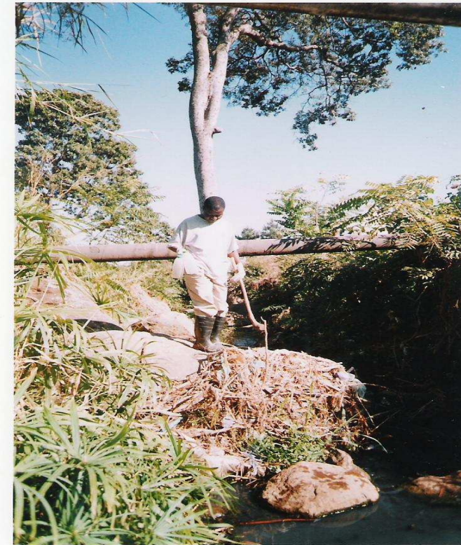
Figure 1.2: A sewer pipe passing over Naperi stream whereby blockages lead to sewage pollution. Residential wastes can be seen collecting on the rocks
